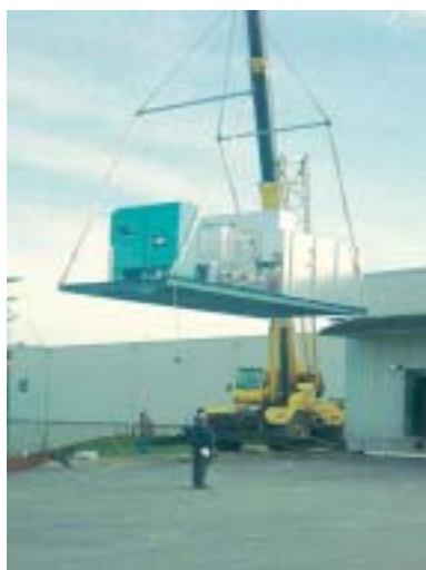
CSM's turnkey services include complete system installations.
