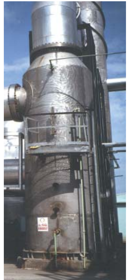
CSM's 45,000 SCFM CatOx at a Taiwan based PTA plant uses this stainless steel water seal for pressure relief.
