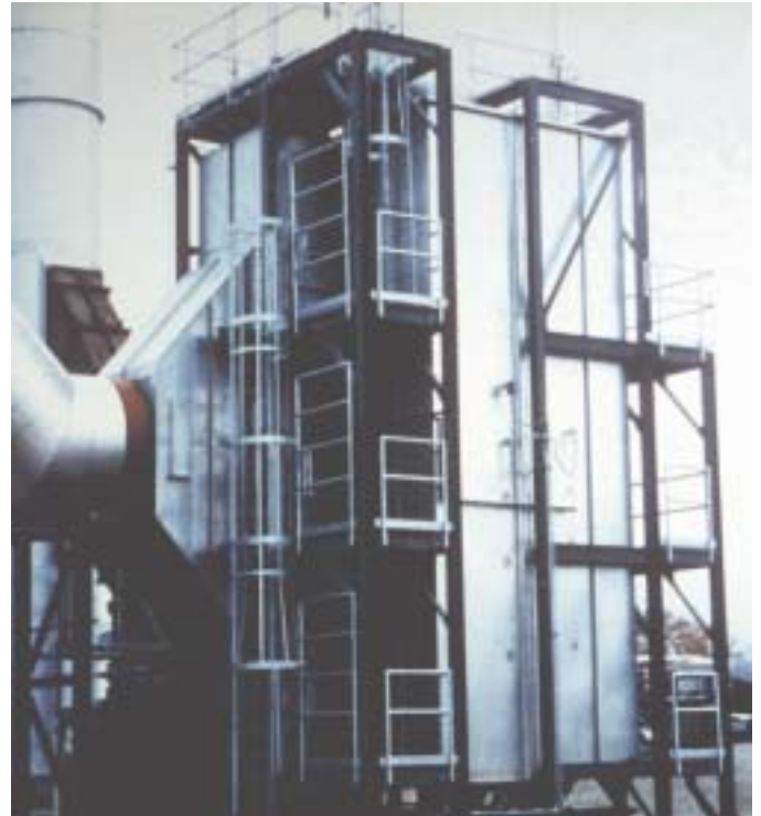
This 60,000 SCFM catalytic oxidizer, supplied by CSM for a major PA manufacturer, was installed in 1991, and currently operates destroying 98% of CO and VOC.
