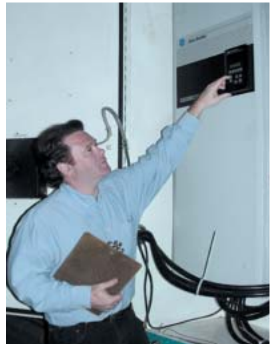
System startup and training, while your plant is in production, assure economic operation and reliable system performance.
