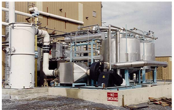
3,300 CFM Skid Mounted ADSOLV Pentane Recovery System with inlet HCl Scrubber - Styrofoam intermediate Manufacturing
